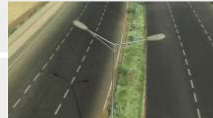
STREET LIGHTS INSTALLED
